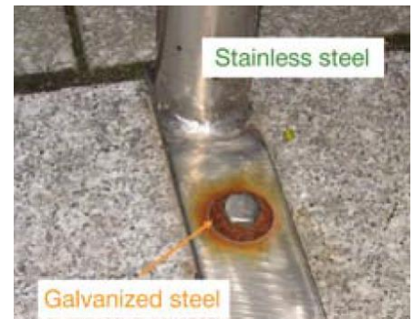
This is a typical case of contact corrosion. Zinc-plated carbon steel (washer) and stainless steel (screw and part) were used together. The surface area of the more noble metal – the stainless steel – is larger, causing strong corrosion of the washer.
