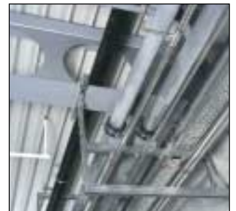
MN system structure on steel beams
