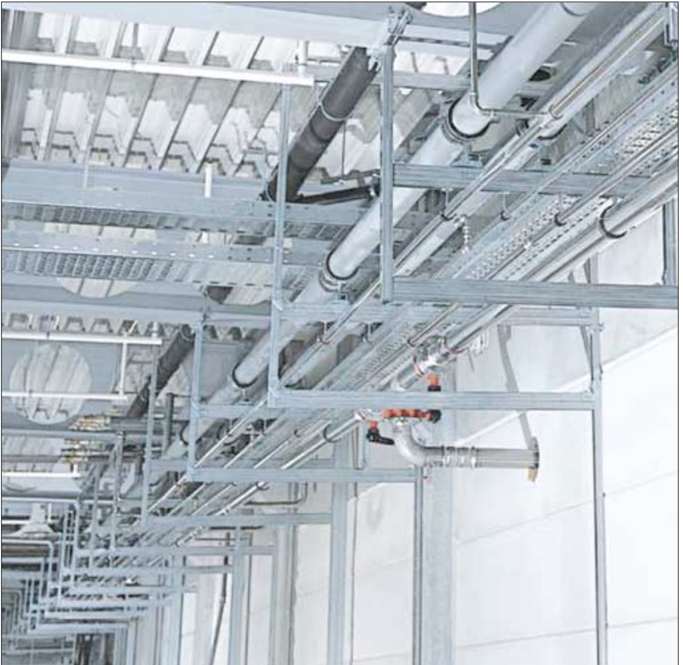
Trend in pipeline installation: Modular pipe run systems for various process lines
